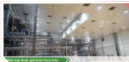
Greenpan panels at the Coca-Cola factory
